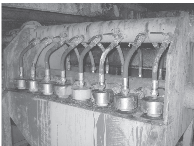
FIGURE 3. The battery of hydrocyclones in MZ-technology.
